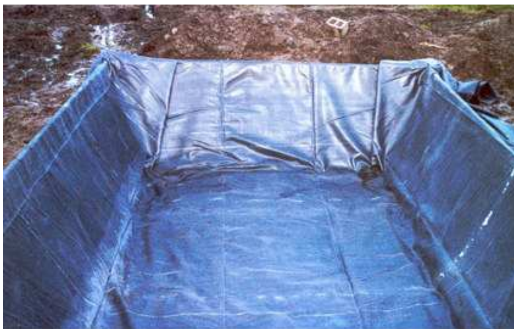
Figure 5: Example of installed constructed wetland liner before filling with gravel media. In this case the liner has been attached to a treated timber frame around the wetland margin. Alternatively it may be anchored to 20 cm depth into the ground via a shallow trench. A water tightness test needs to be carried out when the inlet and outlet pipe connections through the liner have been fitted. (Photo credit: Rob Van Deun, Geel, Belgium)
