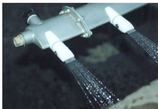
Figure 2. Thru Valve Boom with nozzles orientated horizontally into the air stream.
