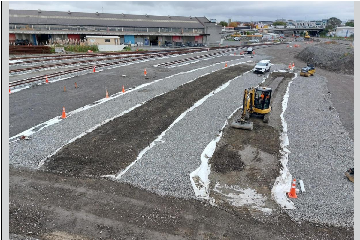
Reuse of fill in the formation of the new rail lines reconfiguration, specifically as backfilling between the tracks, rails, and sleepers and within an electrical line trench, and compacted to meet geotechnical requirements. Geotextile is used to delineate fill, which is then covered with gravel of grade AP20. (Case study provided by Regan Knapp, HAIL Environment)
