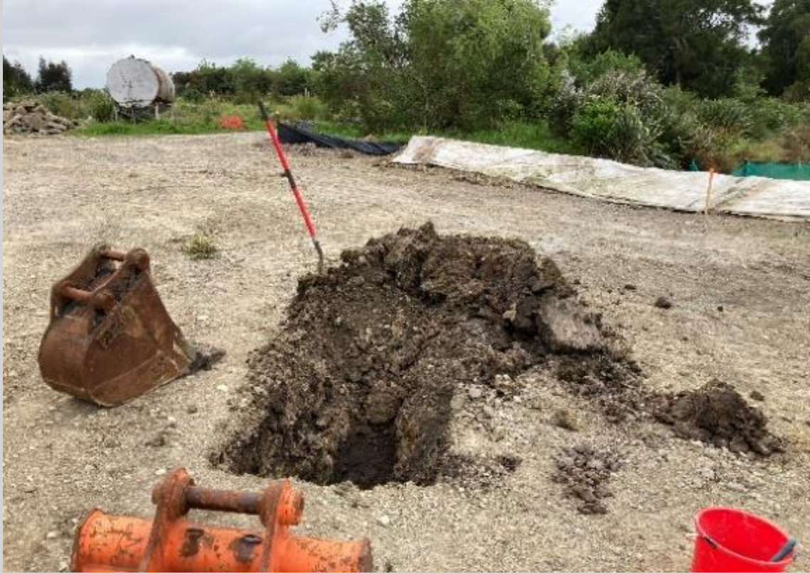
Site soil investigation to determine reuse potential. (Case study provided by Rod Lidgard, PDP Limited)
